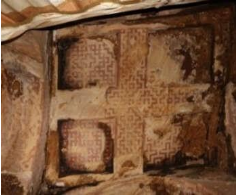
Fig. 9 image showing deteriorating decorated ceiling
