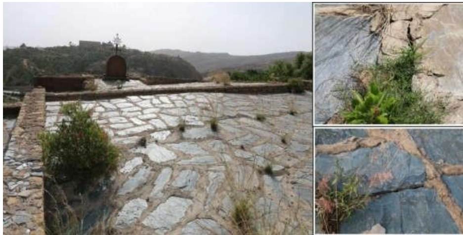
Fig. 6 image showing outcropping grass over the Flagstone roofing
