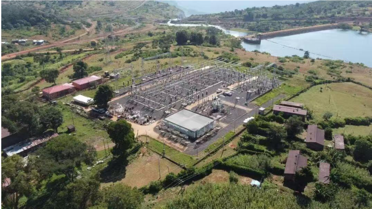
Figure 1-1: Finchaa-II 230 kV Substation Project
