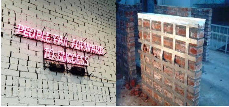
Figure 1-6: wall panel failure
