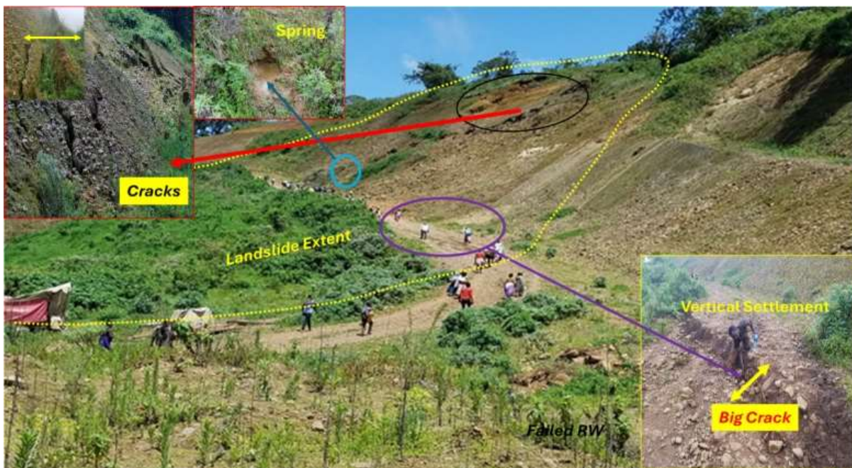
Figure 43: Slope failure with big open cracks on top scarp and springs at slope toe along VH1 at Km 52+200, indicating active landslide with current traffic inaccessibility (Photo taken in August 2021).
