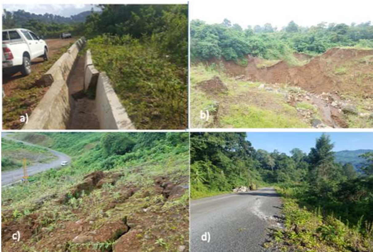
Figure 1: Damage along Bonga–Felegeselam road, showing (a) distorted side ditch, (b) gully erosion, (c) tension cracks, and (d) asphalt differential settlement
