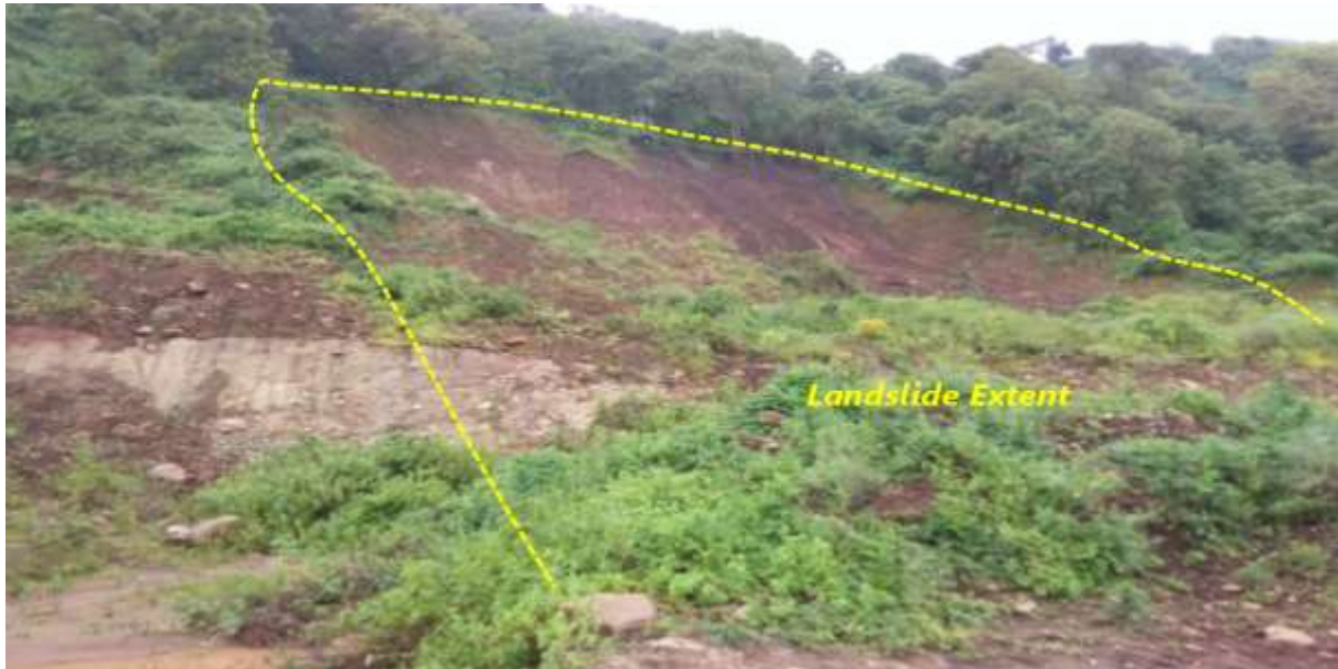
Figure 44: Old debris flow overflowing and cracks on the main scarp along VH2 at Km 53+180, with current road blockage due to active landslide (Photo taken in August, 2021).
