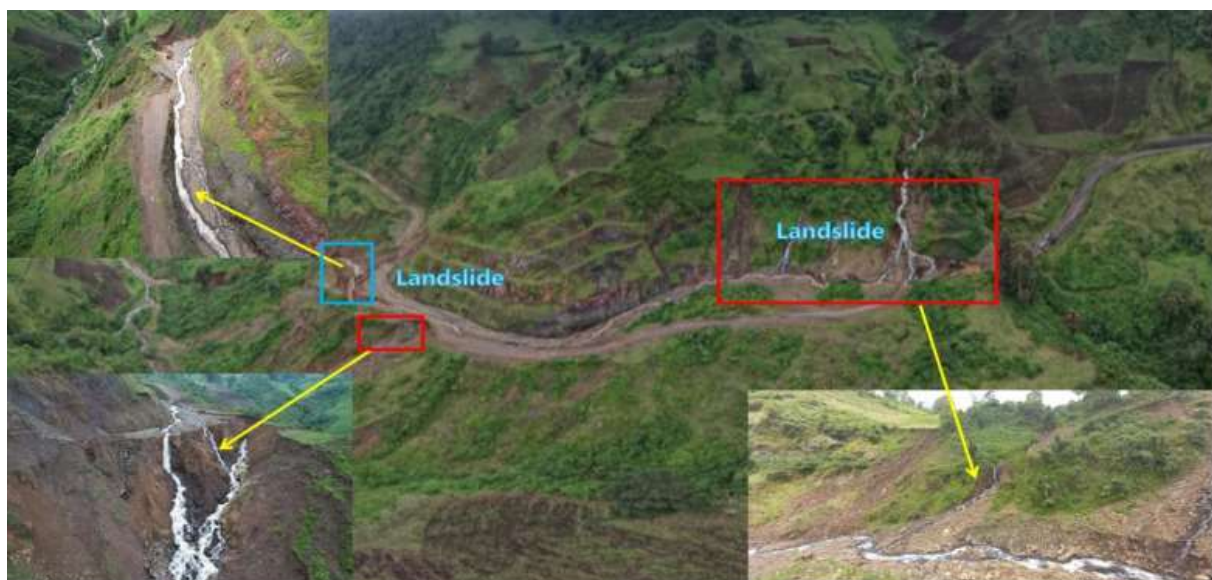
Figure 46: Soil erosion on the face of the back slope and scouring due to roadside erosion and streams along VH4 at Km 65+620, showing significant surface degradation (Photo taken in August 2021).
