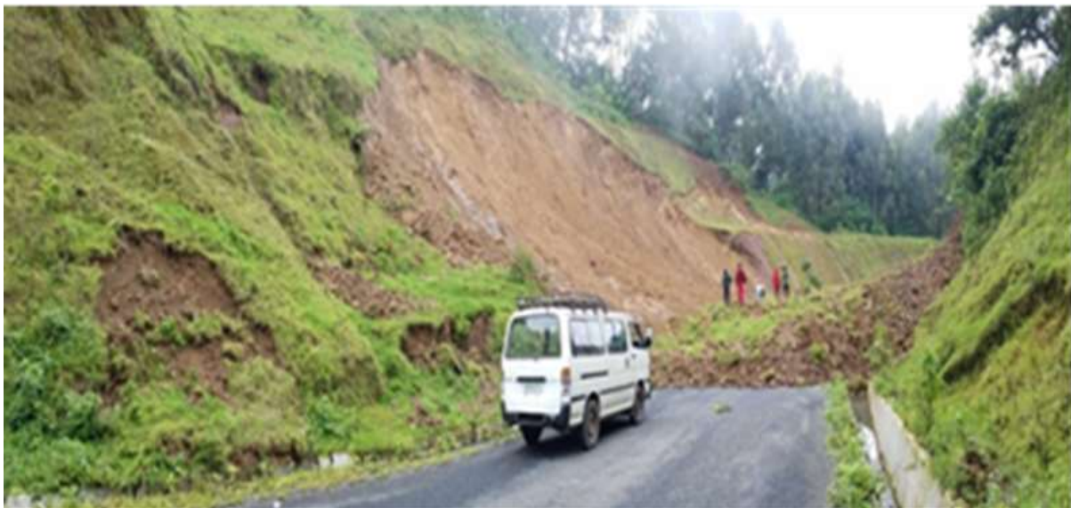
Figure 2: Debris flow blocks Bonga–Felegeselam road near Km 17+340, triggered by heavy rainfall, covering the asphalt.
