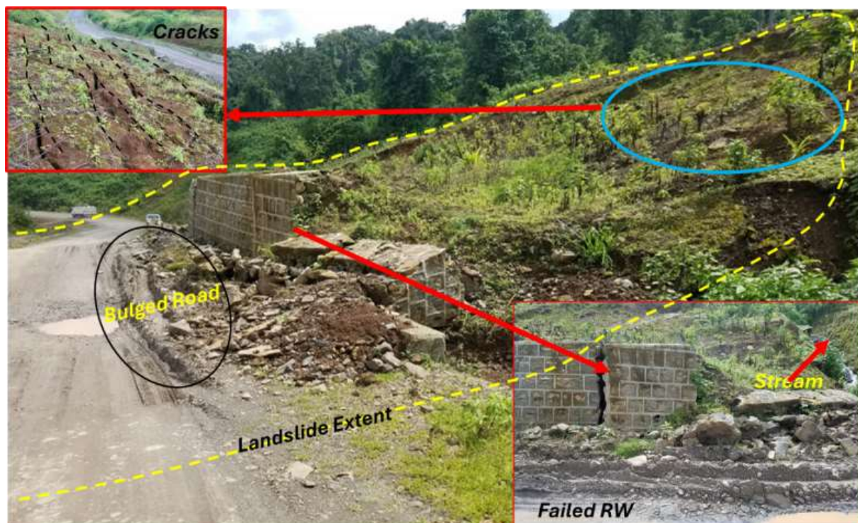
Figure 39: Photo showing failed retaining wall, tension cracks, and bulged road along M1 at Km 20+470, illustrating structural failure and ground deformation (Photo taken in August 2021).
