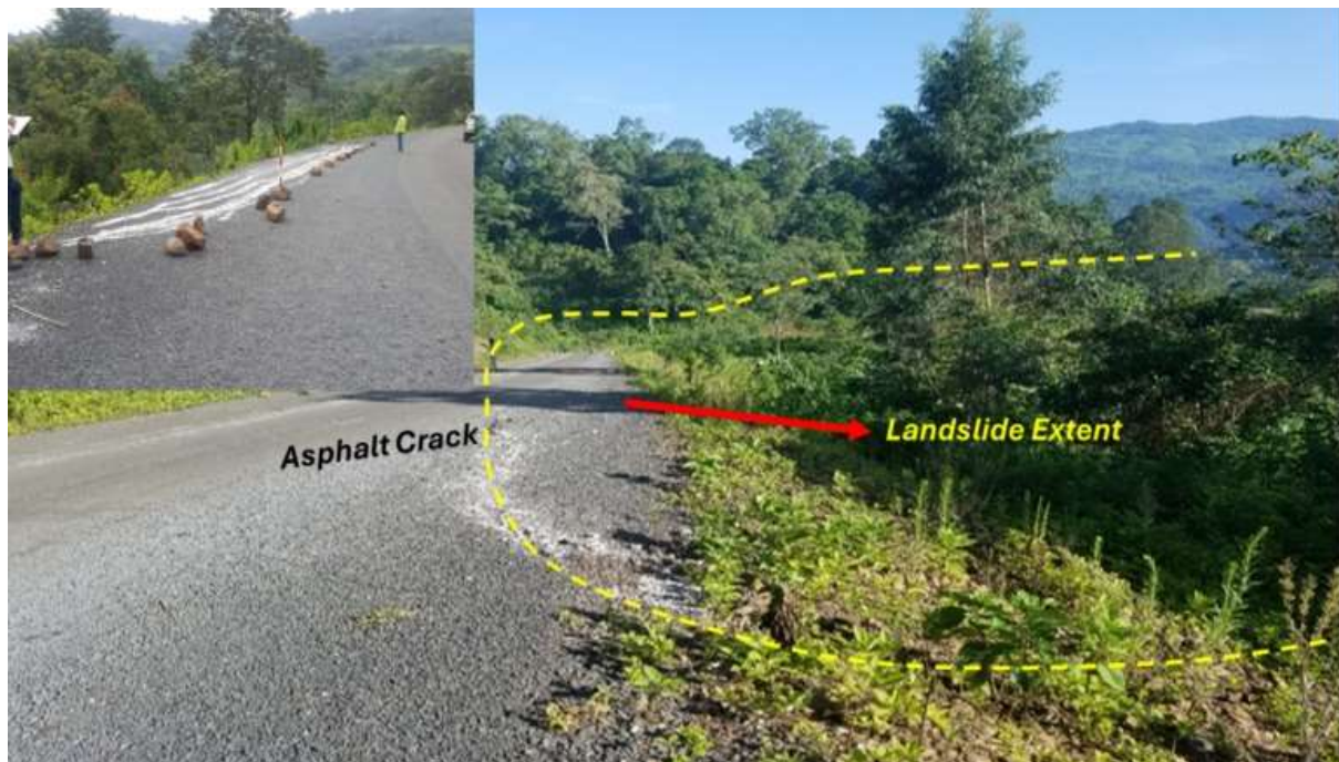
Figure 40: Asphalt settlement over high fill section with longitudinal cracks along M2 at Km 35+220, indicating pavement distress (Photo taken in August 2021).
