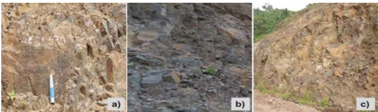
Figure 14: Middle Basalt Flows (TV5) at Km 63+600. Slightly weathered basalt exposure with random jointing observed along the left-hand side of the road.
