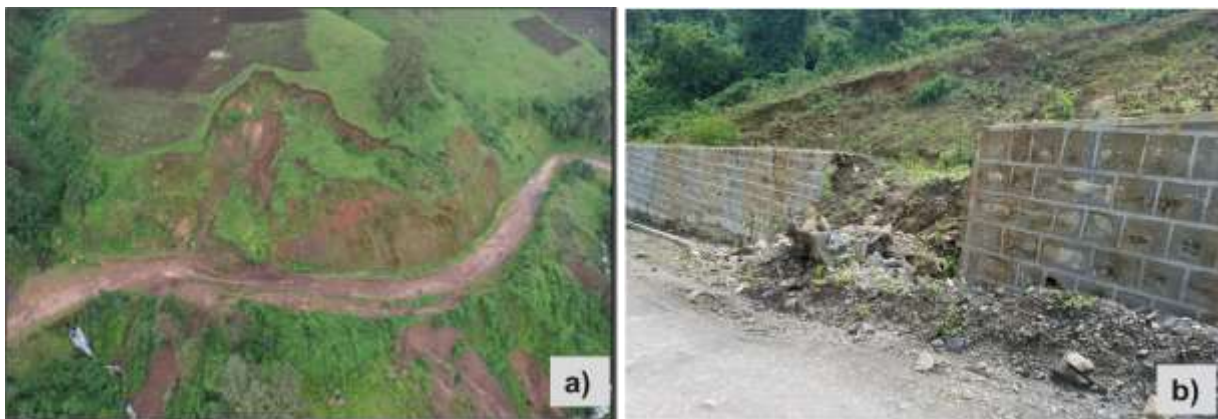
Figure 20: Overview of observed landslides in the study area. (a) general view of rotational landslides, triggered by road cutting, impacting the roadway, (b) additional view of rotational landslide activity, that damaged retaining structure. (Photographs were taken in August 2021).
