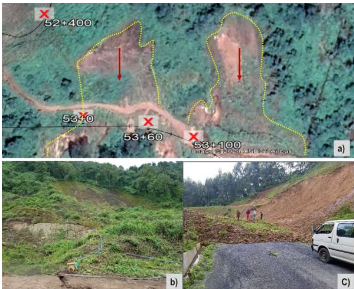
Figure 19: Overview of debris and earth flows from a steep hillside near Migra down to the road. (a) Satellite view from google earth; (b) ground photo showing debris flow paths; and (c) Earth/mud flows along the road cut slope blocking the road (Photographs taken in August 2021).
