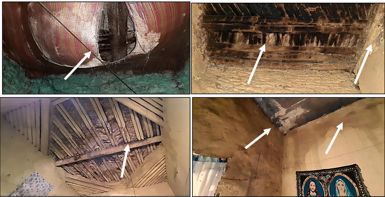
Picture 14: Leakage (Seepage) Damages of Blata Tsegay Mansion House. Field Survey, 2020.
