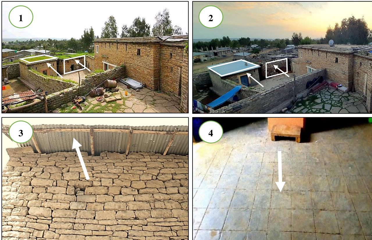
Picture 25: Use of Inappropriate Materials, on Assefa Tedla Mansion (Pic 1, 2, 4) and Blata Tsegay Mansion (Pic 3). (Pic. 1, Sources, Ashu Pictures, 2012 G.C), and Field Survey, 2020.
