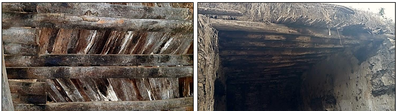
Picture 15: Moisture and Dampness Damage, Case Study (Compound Three Kitchen Ceiling), and Kebele 14 Random Hidmo Ceiling. Field Survey, 2020.
