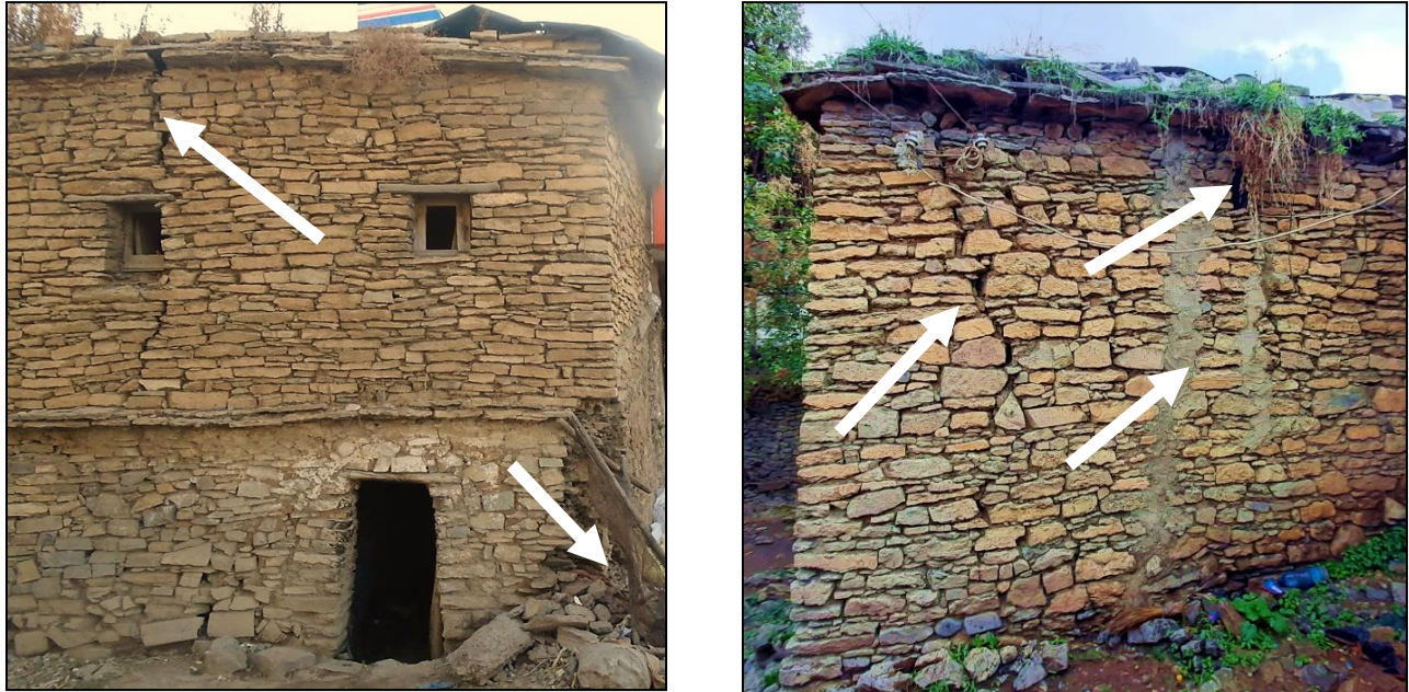
Picture 13: Earthquake Damages, a Hidmo Houses in Kebele14. Field Survey, 2020.
