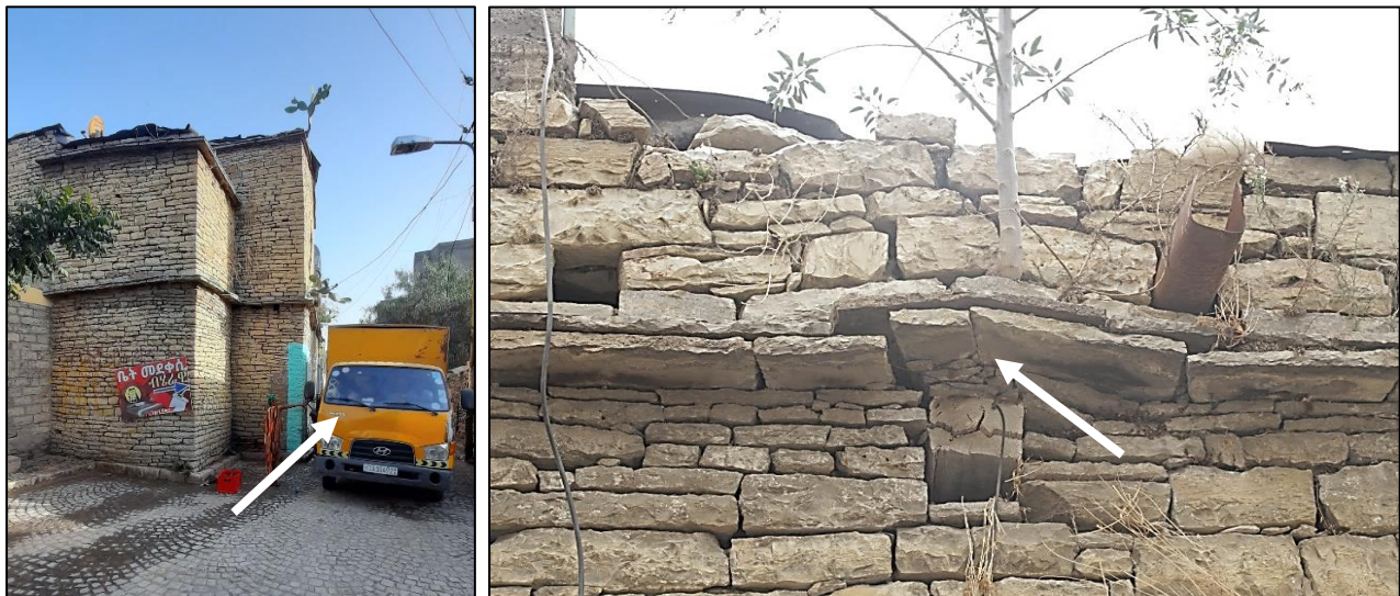
Picture 22: Passing Heavy Vehicles Along the Way that Caused Vibration on Blata Tsegay Mansion. Field Survey, 2020.
