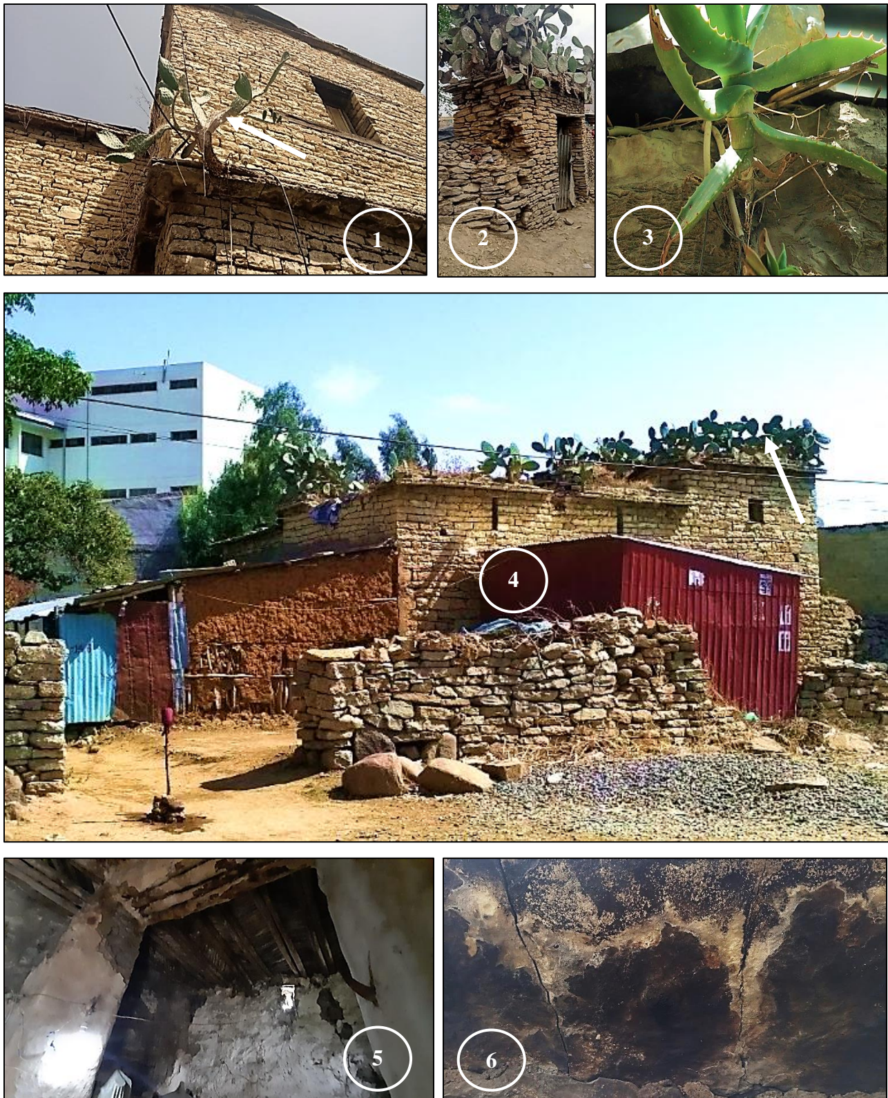
Picture 17: Damage Due to Trees and Vegetation Growing in the Case of Kebele 14, (Pic. 1, 2, 3), and (Pic. 4, in Aynalem Area). Due to Temperature Fluctuations also, Shows (Pic.5 and 6, in Aynalem Area). Field Survey, 2020.
