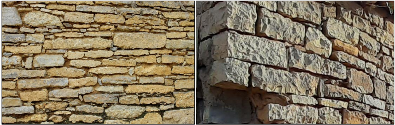
Picture 50: Typically Coursed Rubble Masonry (CRM), and Coursed Square Masonry (CSM), With MW Technique of the Compounds. Field Survey, 2020.
