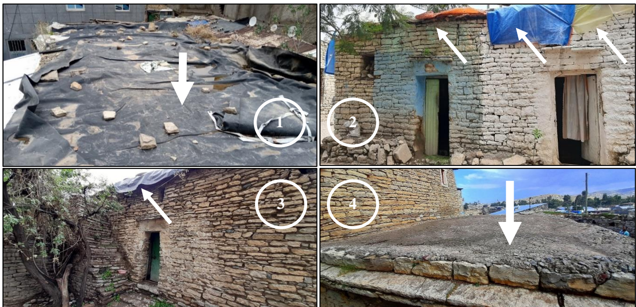
Picture 12: Rain Damages of Hidmo Houses in Kebele 14 (Pic. 1, 2, 3, 4, 5) and (Pic. 6, Aynalem). Field Survey, 2020.
