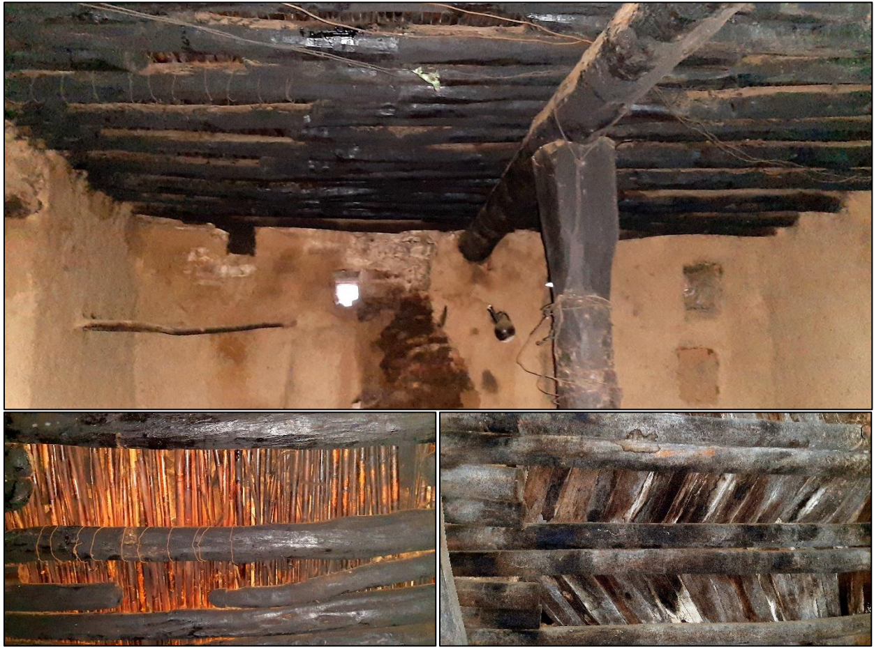
Picture 52: Rain Leakage and Smoke Damages of the Kitchen Ceilings. Field Survey, 2020.
