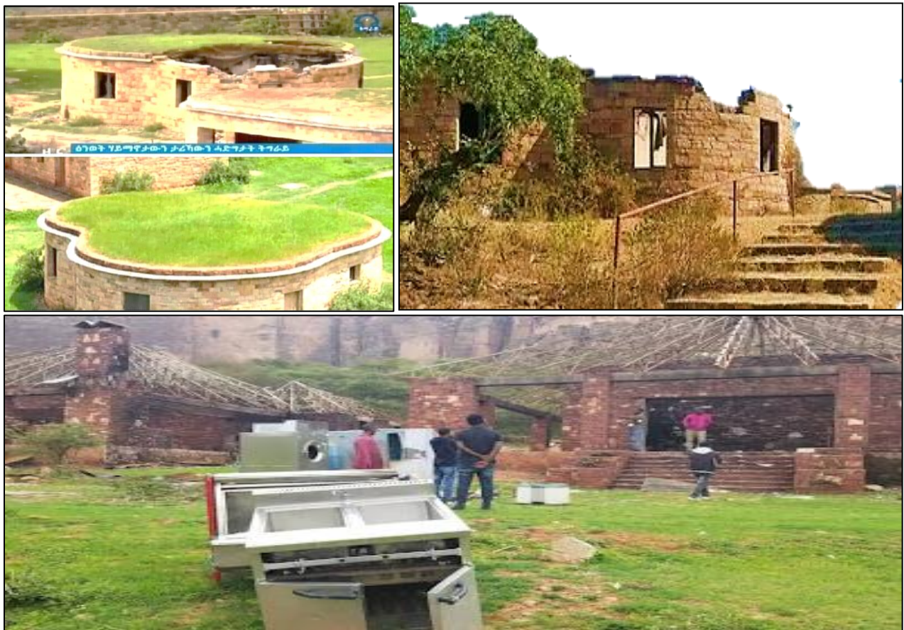
Picture 45: Gheralta Lodge Damage, Hawzen, Tigray. Pic. Tigray TV, 2022 G.C. and Showed the Destruction of the Newly-Built Gheralta Kurifutu Sabian Lodge. Tghat.Com Respectively.
