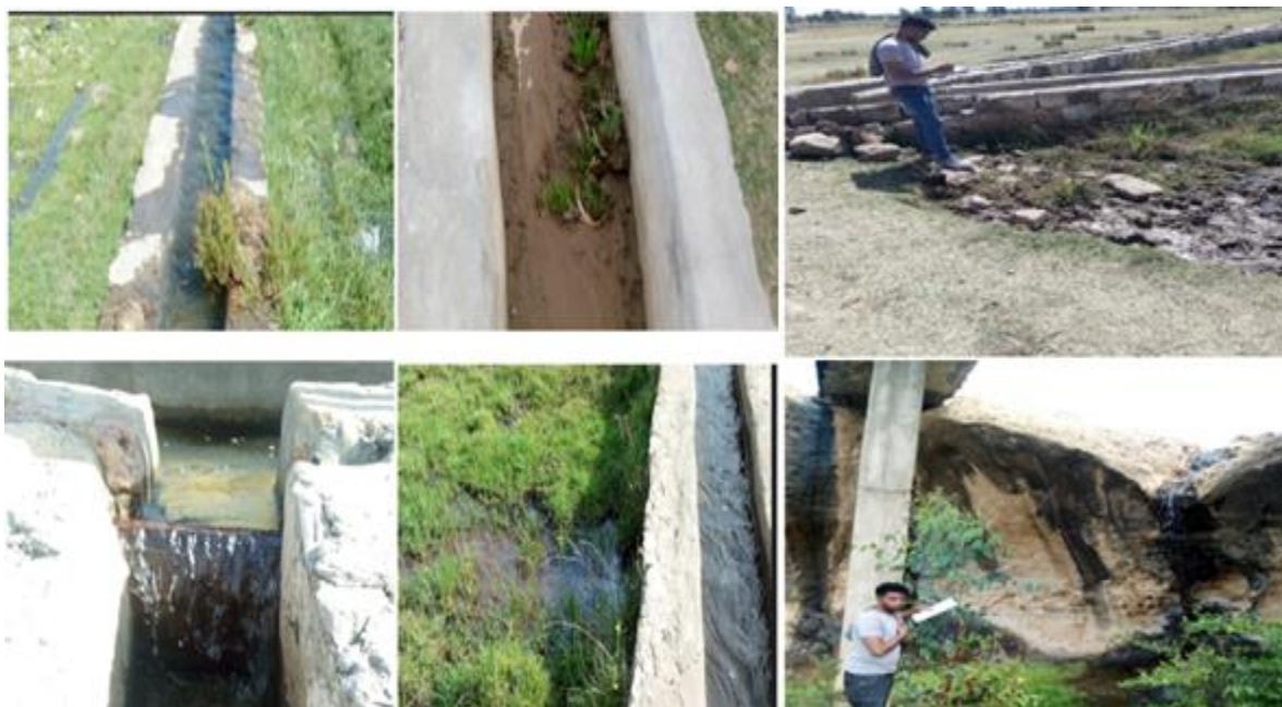
Figure 4-1: Current status of physical infrastructures in the Hangoda irrigation scheme
