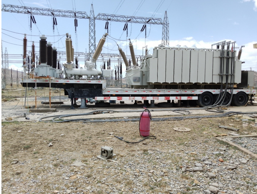
Figure 1.4: Mobile substation of Mekelle substation
