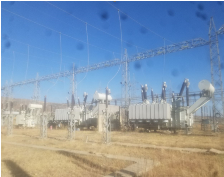
Figure 1.2: Outdoor (Switchyard) of Mekelle substation
